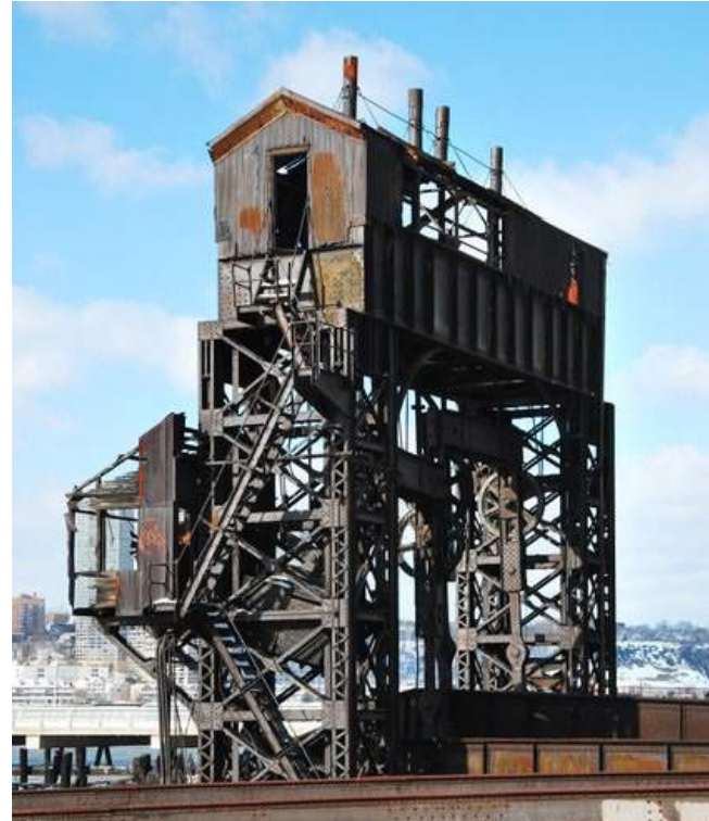
Abandoned 69th Street Transfer Bridge
