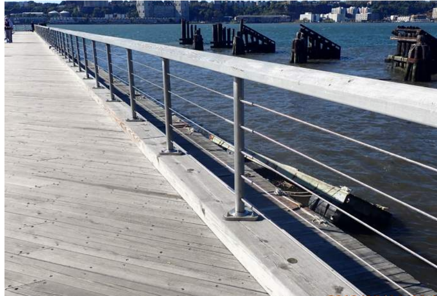
A-Dock Pipe/ Cable Searail
