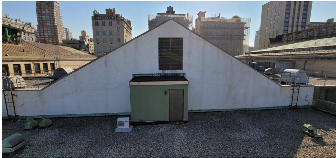
PHOTO OF WEST FACING GABLE WALL. EXISTING STUCCO PROPOSED TO BE REPAIRED AND CLAD WITH INSULATION AND METAL PANEL RAINSCREEN CLADDING
