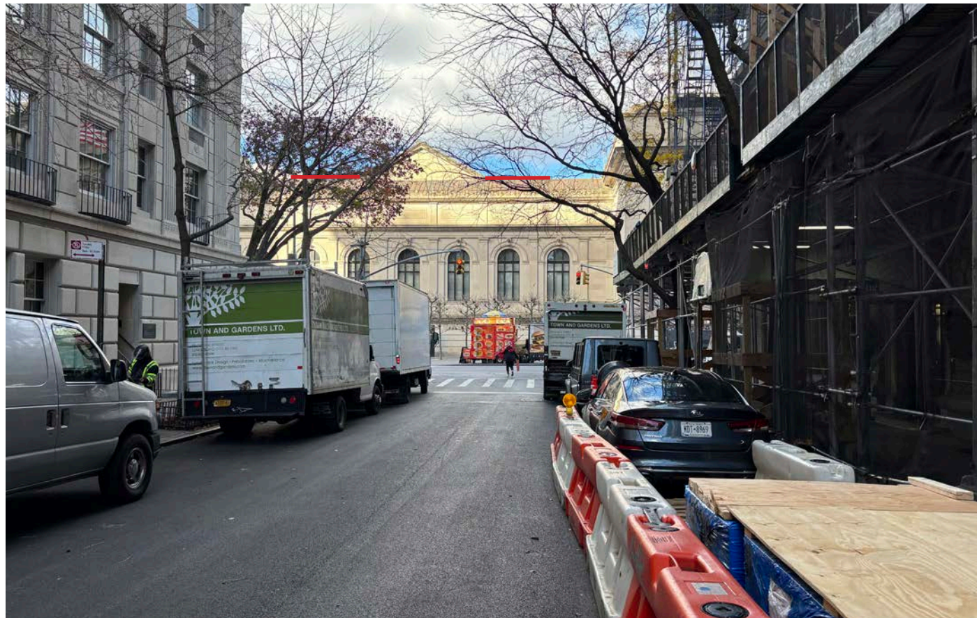
MONTAGE VIEW 2 - TOP EDGE OF SCREEN WALL BECOMES VISIBLE (RIGHT OF PEDIMENT) HIGHLIGHTED WITH RED LINE RESTORATION OF THE 83RD STREET ENTRANCE AND NORTHSIDE CHILLER PLANT REPLACEMENT
