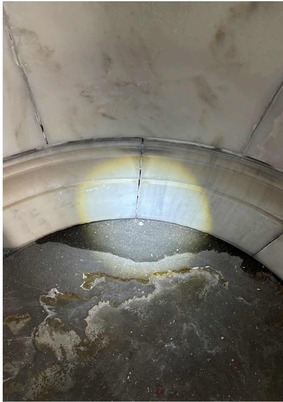
2— Evidence of water intrusion & damage
