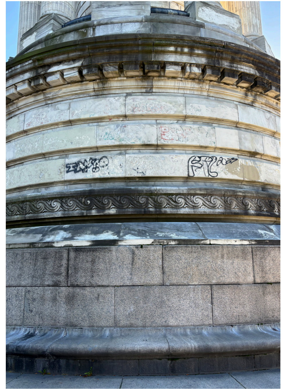
3— Deterioration of masonry elements
